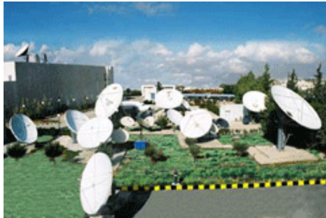
The antenna farm of the Jordan Media Center in Amman. (photo courtesy of Jordan Media Center)
